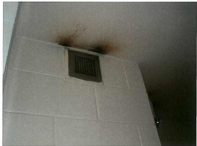
DETENTION FACILITY – HVAC. from Cell Interior
