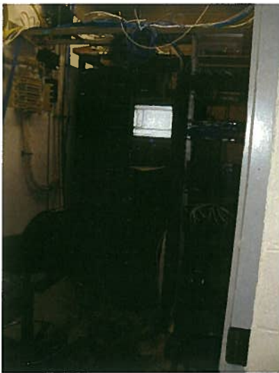
DETENTION FACILITY - Security Electronics Closet
