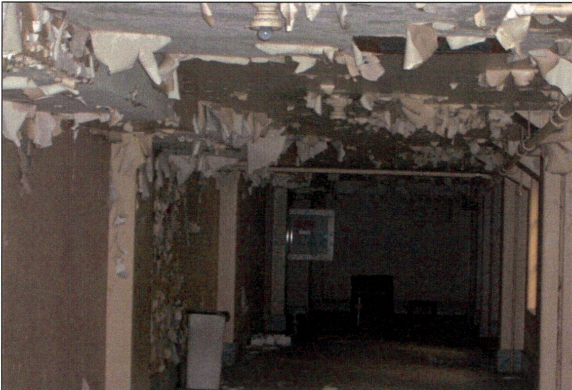
Photograph 8: Typical flaking lead-based paint
