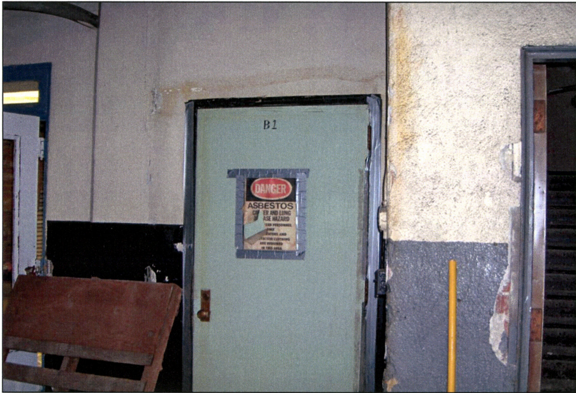
Photograph 15: Basement room containing bagged asbestos material
