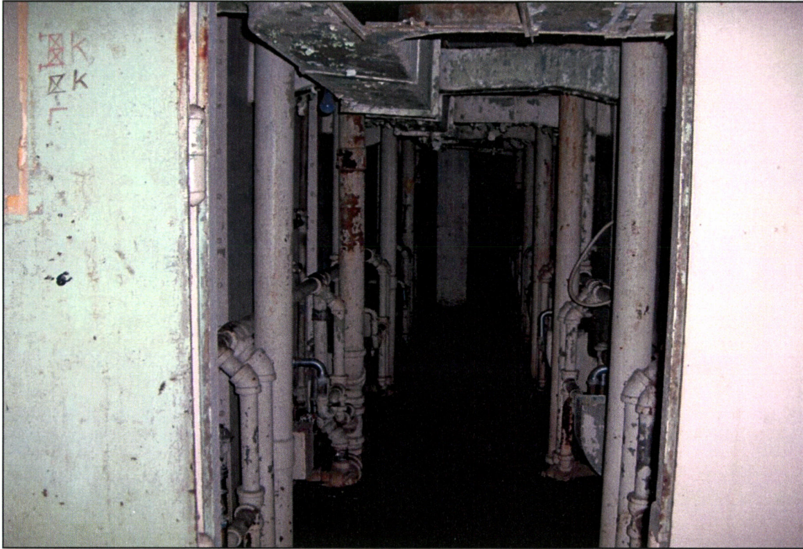
Photograph 7: Typical pipe chase between prison cells with asbestos containing insulation
