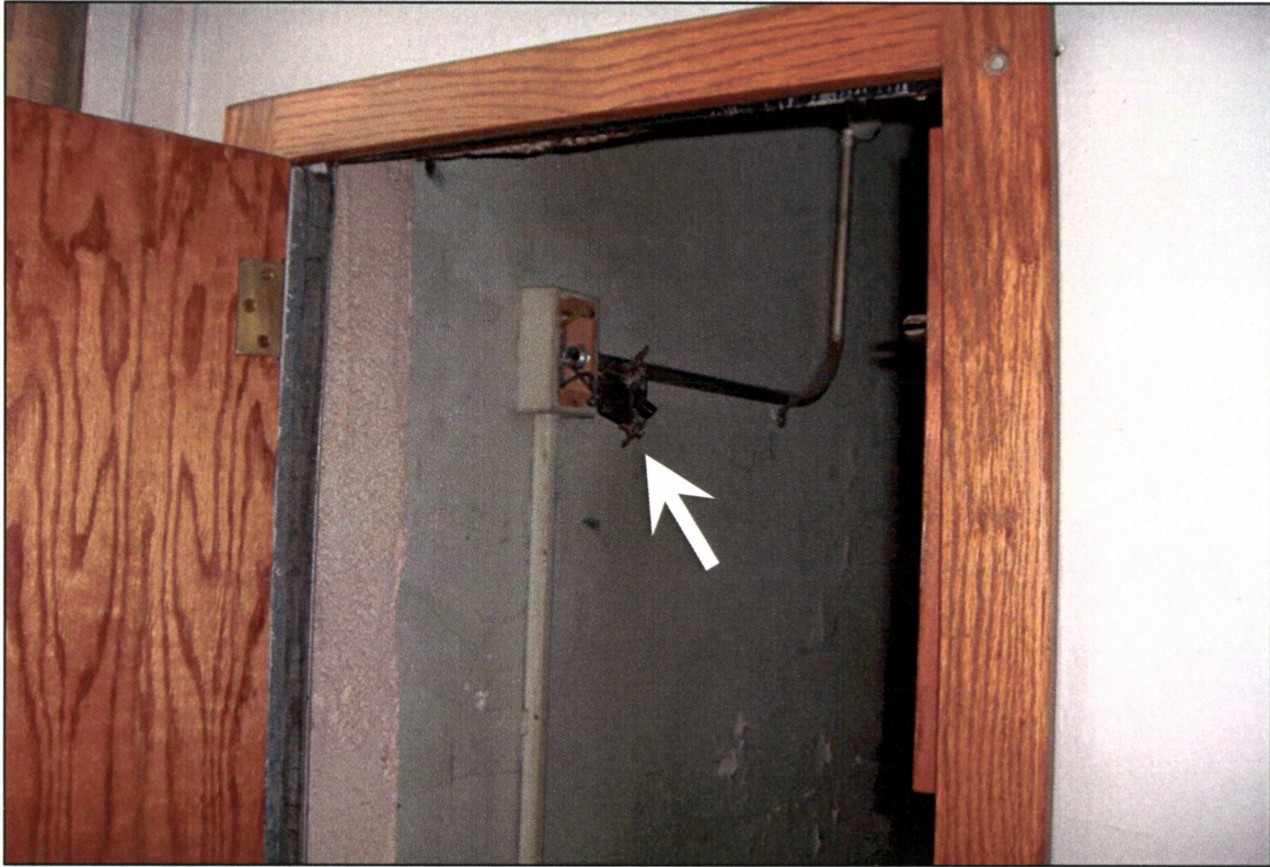
Photograph 13: Typical mercury switch
