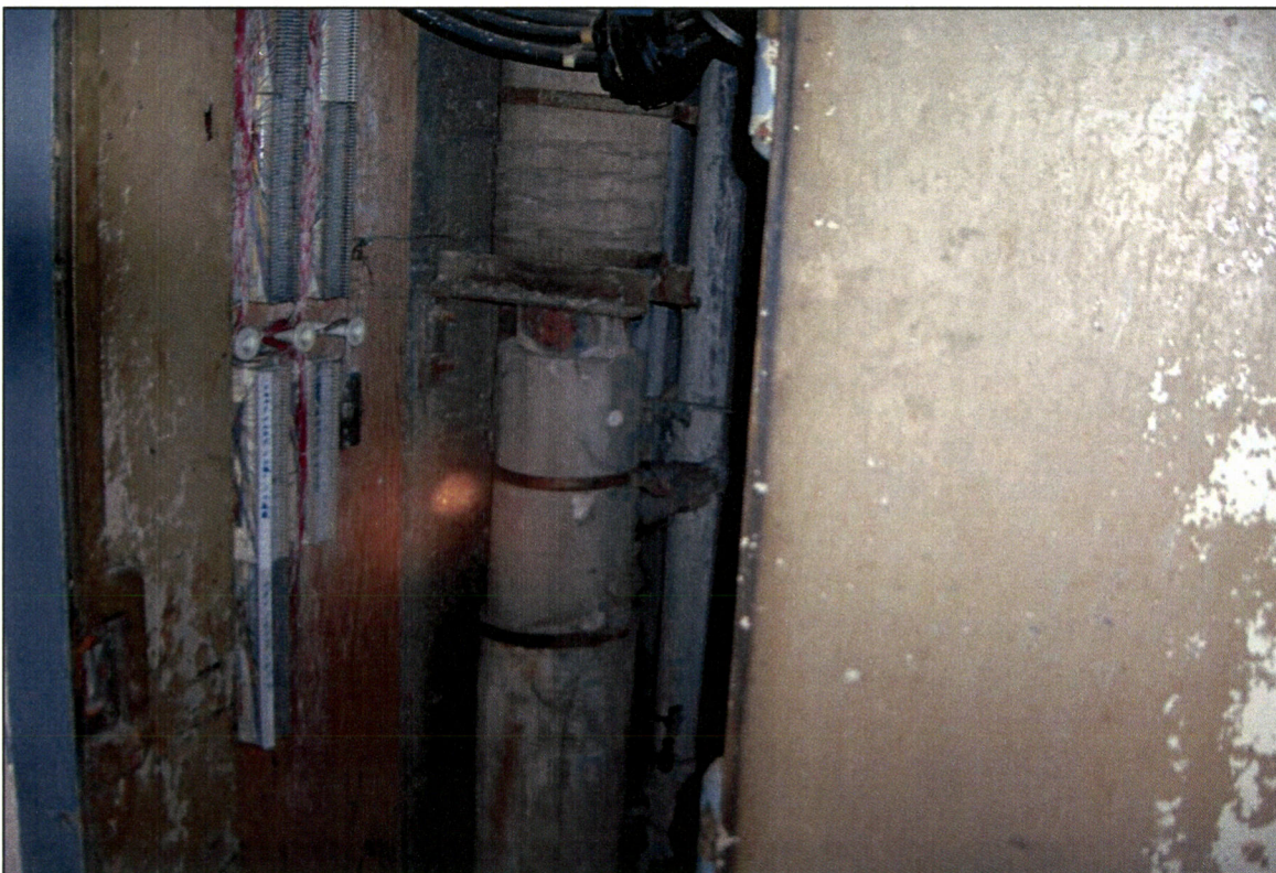
Photograph 6: Typical vertical piping with asbestos containing insulation
