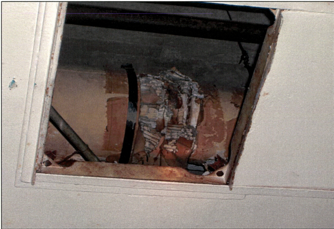
Photograph 4: Typical asbestos containing pipe insulation
