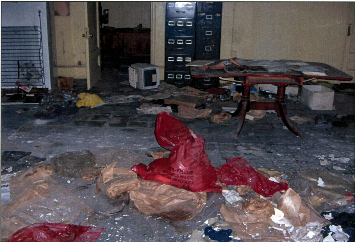
Photograph 14: Biohazard bags in room 100 on 1 st floor
