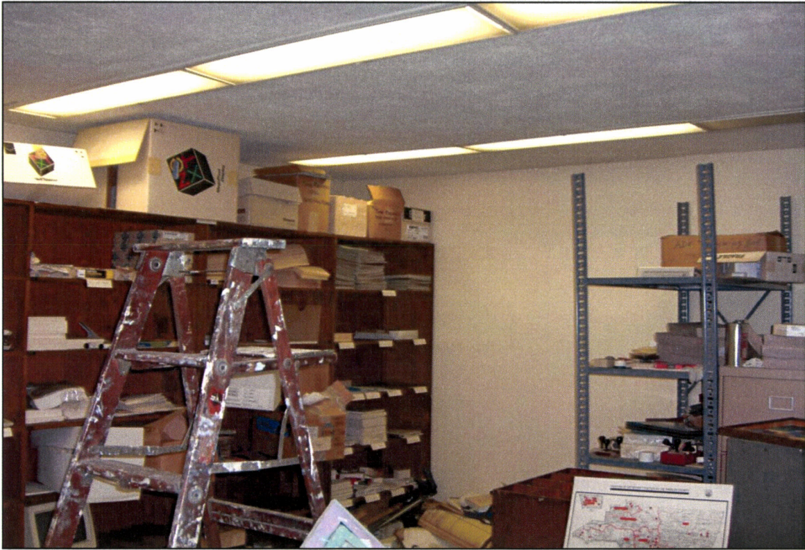
Photograph 11: Typical fluorescent light fixtures
