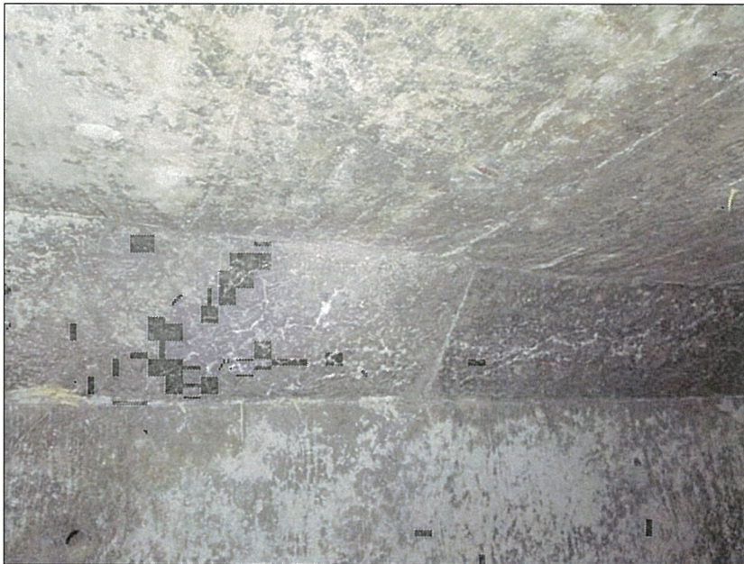
PHOTO 14: CEILING AND TOP CORNER OF WEST WALL OF EAST BAY AT STATION 55.
