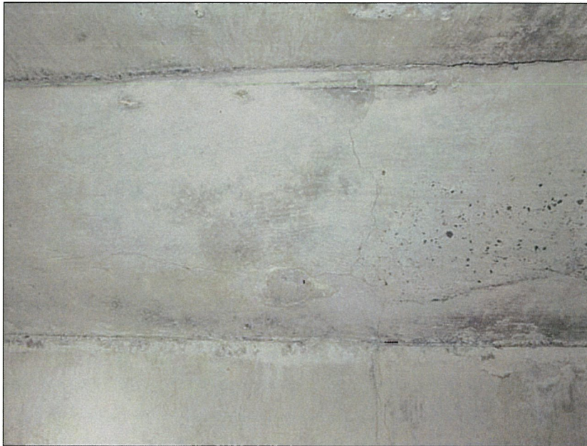
PHOTO 6: TOP CORNER OF WEST WALL OF WEST BAY AT STATION 260.
