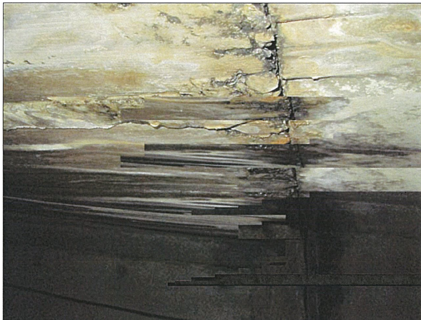
PHOTO 24: LOOKING EAST AT CEILING OF CULVERT 2 AT STATION 610.
