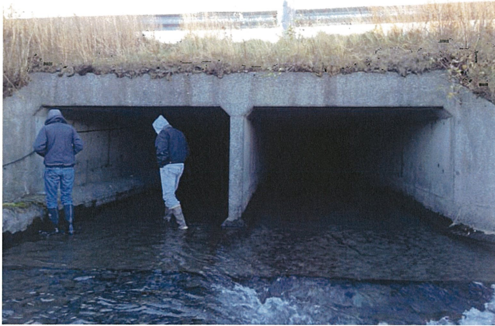
Airport culvert outlet—note concrete encased pressure sewer in culvert on left side of photo. Photograph looking upstream
