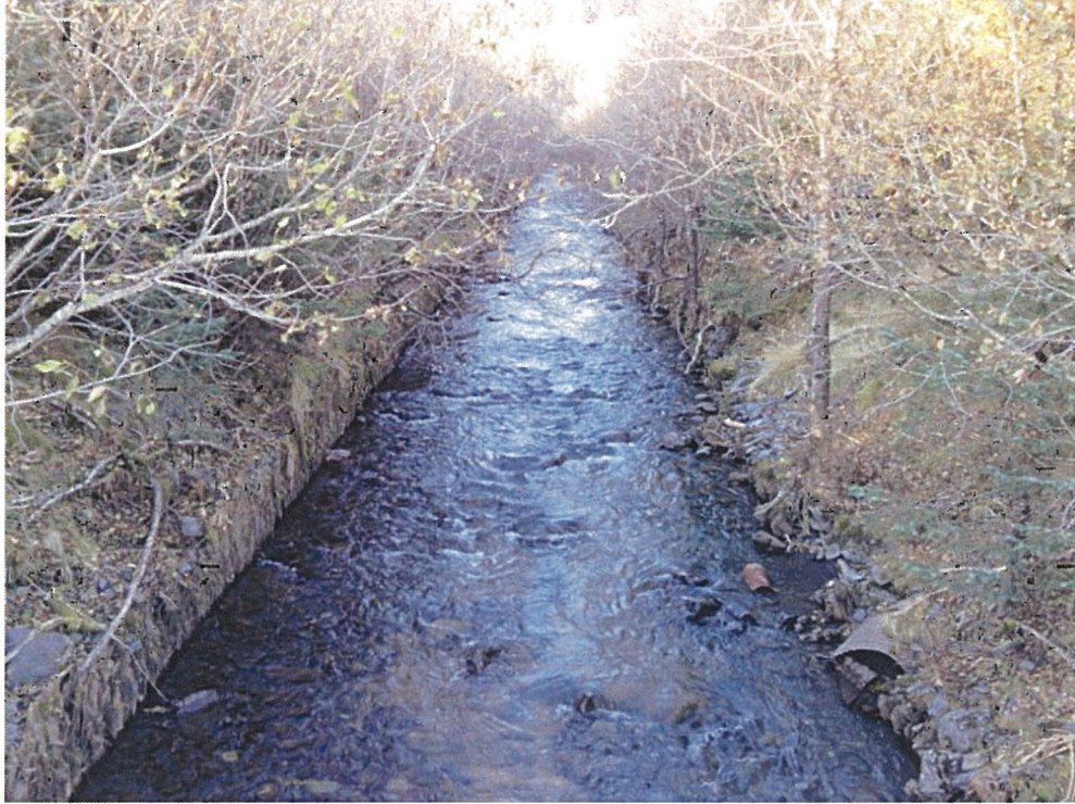
Remnants of relic wooden box culvert between Rezanoff Drive and maintenance road bridge. Photograph looking upstream.
