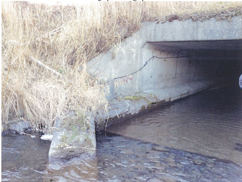
Airport culvert outlet. Detail of concrete encased pressure sewer in culvert. Photograph looking upstream
