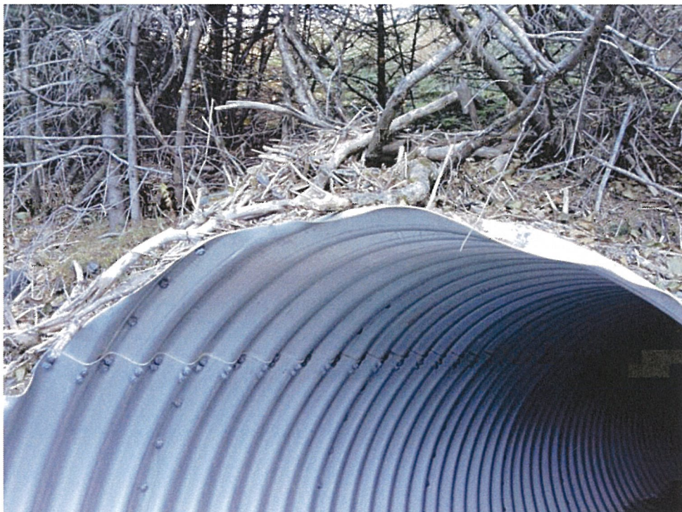
Inlet to Rezanoff Drive 12-foot-diameter aluminum CMP—note flood debris above culvert inlet. Photograph looking downstream.
