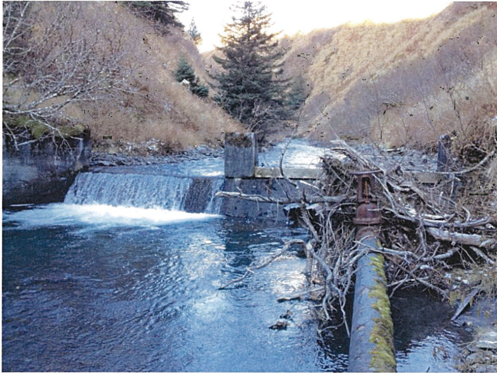
Abandoned concrete dam—note brush debris on valve operator. Stoplog support in center of photo. Photograph looking upstream.
