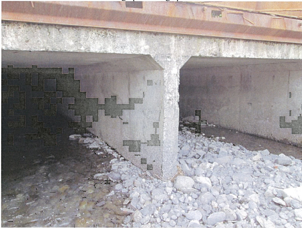
Airport culvert intake—note sharp edges on concrete inlet and gravel in invert. Photograph looking downstream.
