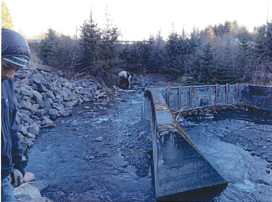
Abandoned concrete inlet structure—note Rezanoff Drive 12-foot-diameter aluminum CMP in background and riprap on left bank. Photograph looking downstream.
