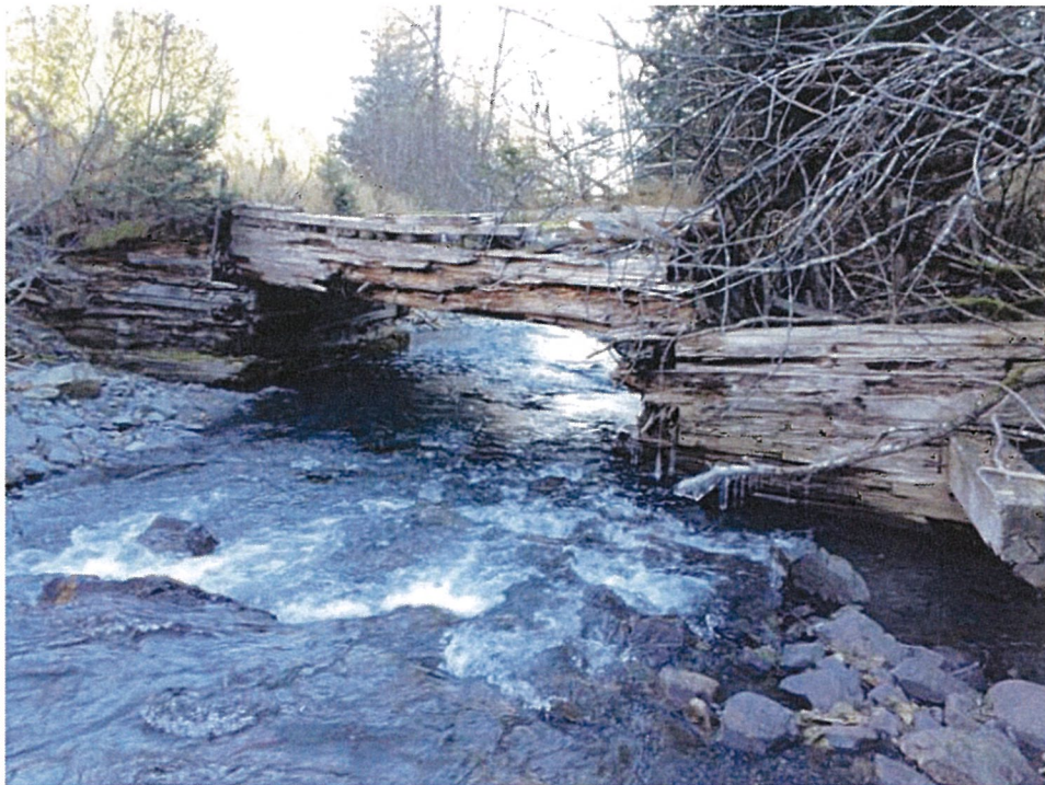
Abandoned wooden bridge Photograph looking downstream. (Post note: Bridge was removed in 2012)
