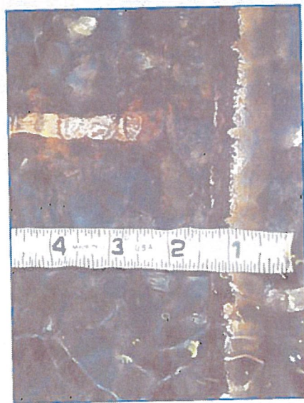
FIGURE 8. Note that longitudinal bars are also exposed in some areas.
