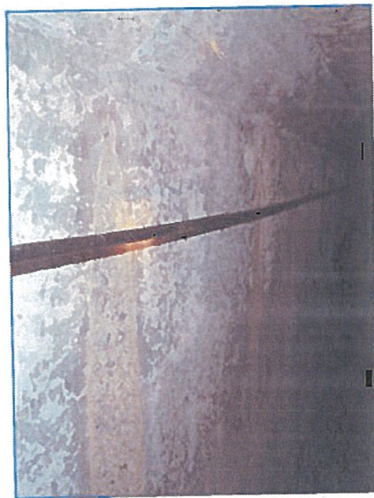
FIGURE 12. Minor seepage and surface damage through form tie holes. Also shown here is an abandoned utility cable that is not in service.
