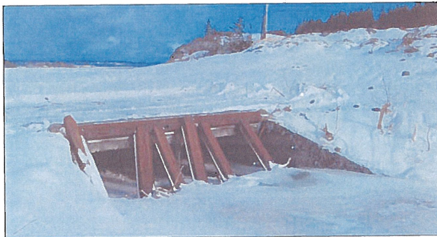
FIGURE 3. The inlet of the Devils Creek Culvert at the Kodiak Airport (March 9, 2010).
