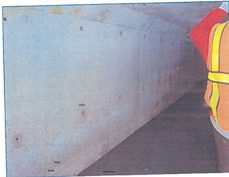
FIGURE 18. Though difficult to see in the photograph, water “stains” on the sides of the culvert are useful indicators of flow depths and recurrence. Shown here are indications that flow depth regularly exceeds the mid-height (form tie) holes.
