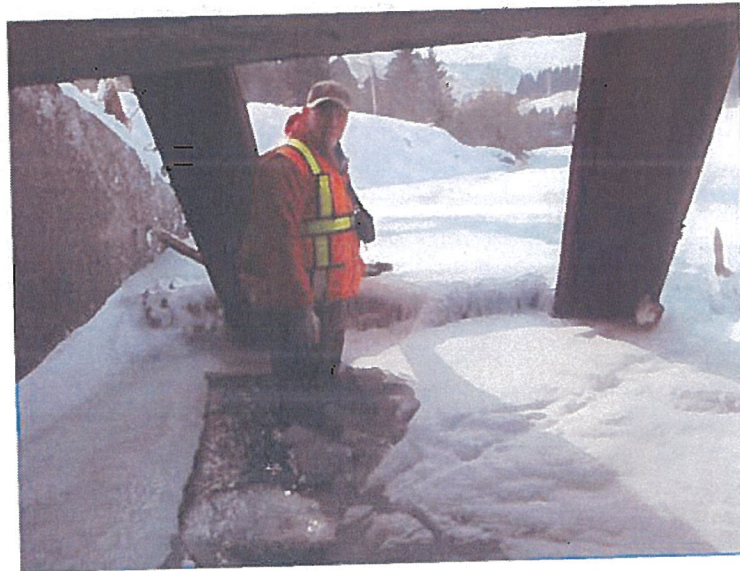
FIGURE 16. A frazil ice terrace at the culvert inlet.
