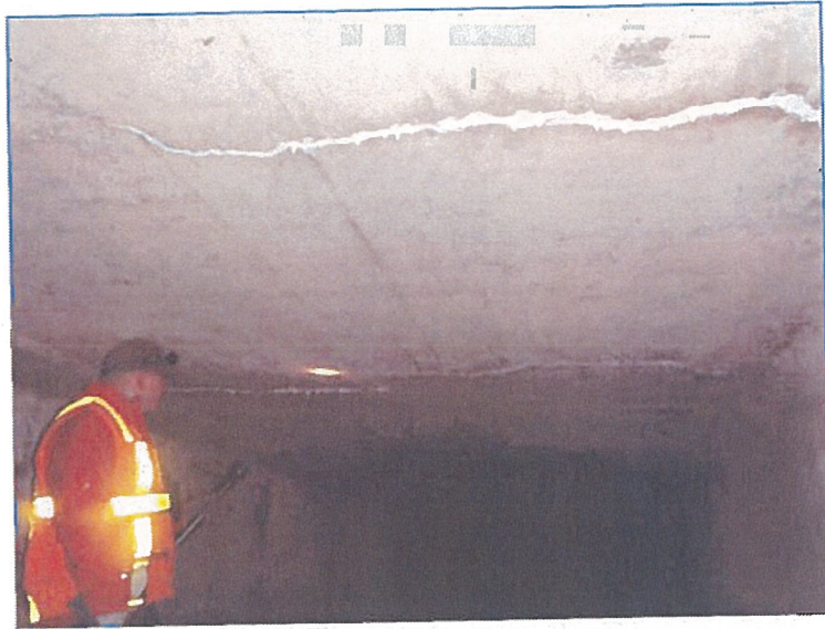
FIGURE 9. Efflorescence evident with cracks.
