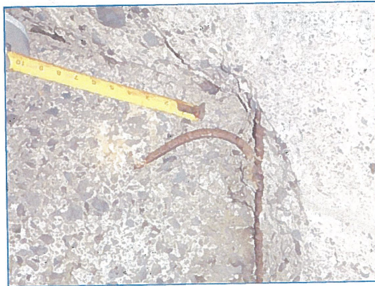
FIGURE 14. Reinforcing steel at the location where the encased utility enters/leaves the box culvert.
