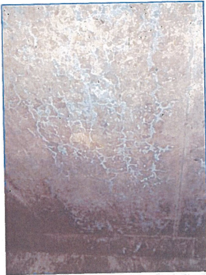
FIGURE 11. "Map cracking" along the top of structure, mostly evident in the upstream 1/3 of the culvert
