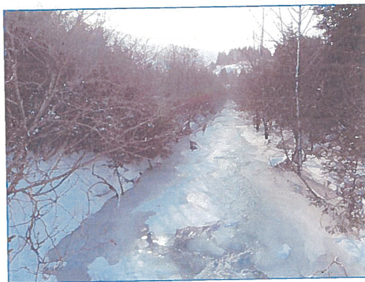
FIGURE 22. View of the channel upstream of the culvert between the M&O access road and the Rezanof Drive culvert.
