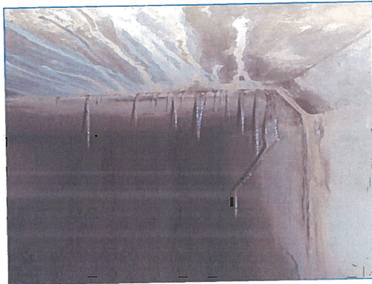
FIGURE 10. Minor seepage (icicles) and efflorescence at a joint.
