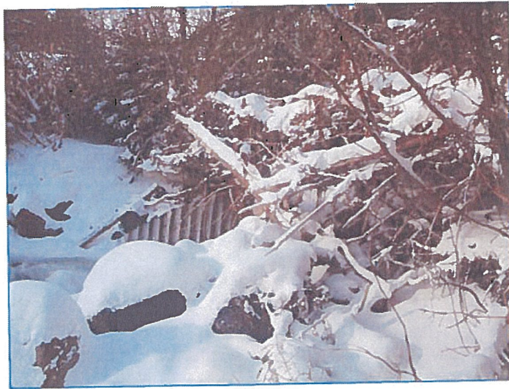
FIGURE 23. Upstream culvert beneath Rezanof Drive with debris accumulation at the inlet.
