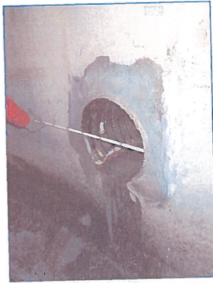
FIGURE 27. An 18-inch corrugated metal pipe entering the river-left barrel approximately 450 ft upstream of the outlet. This corresponds to the drainage swale between the runway and taxiway.
