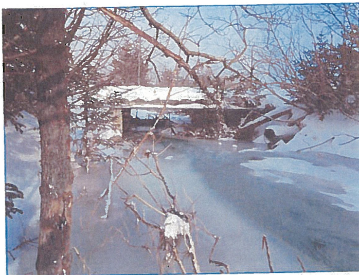
FIGURE 21. Maintenance access road/bridge upstream of the culvert. Note the debris accumulation at the bridge.
