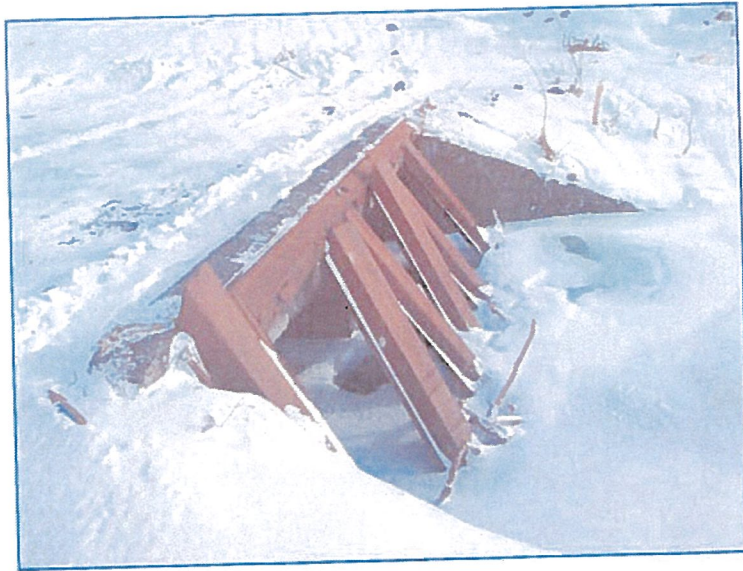
FIGURE 15. "Debris rack" at the culvert inlet with ice accumulation.
