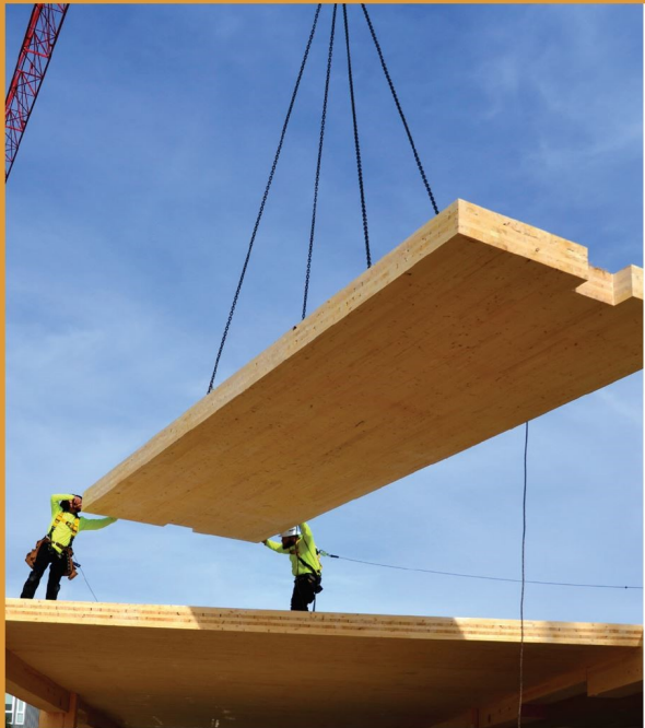
A Carpenter crew assembling the pre-cut cross-laminated timber (CLT) panels at 1 De Haro Street, the first project in San Francisco to use CLT.
